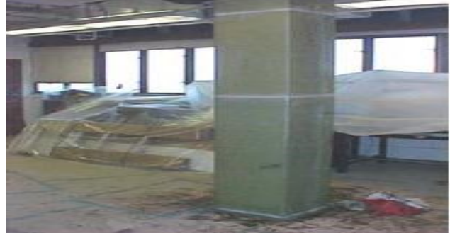
Fig.8: Depict the use of advance composite in the healing of concrete spall on wall ( Chiewanichakorn & Toranzo, 2011 ).
