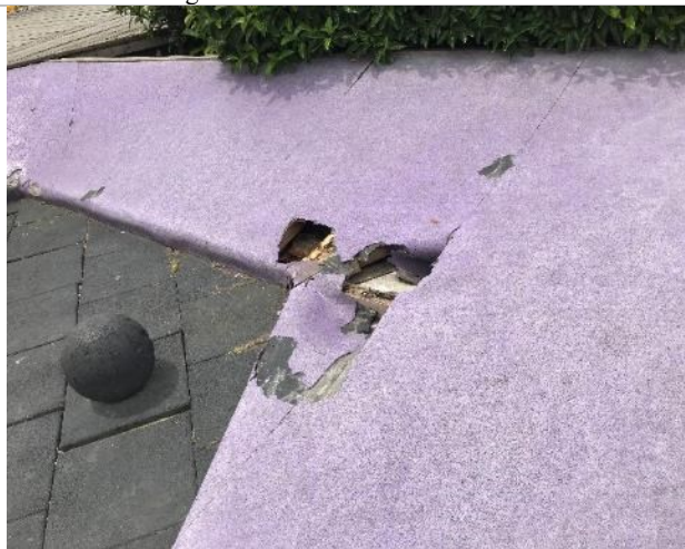
The material in the entertainment corner has deteriorated and is left unmaintained.
