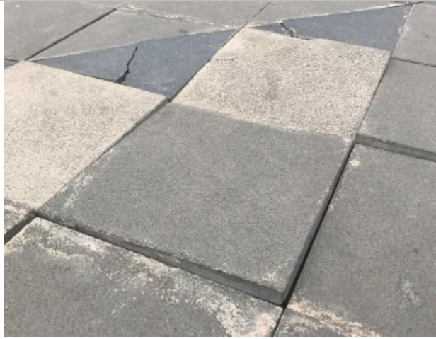
Ground floor tiles are short-lived and of poor quality.
