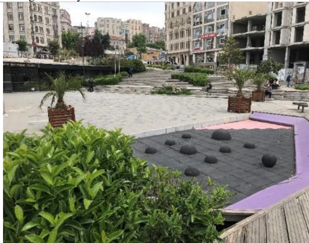
The entertainment corner in the Şişhane park is unusable because of damage to the used materials.
